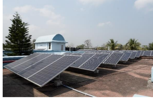
Figure 2.16. Solar Panel at the rooftop of Administration building
